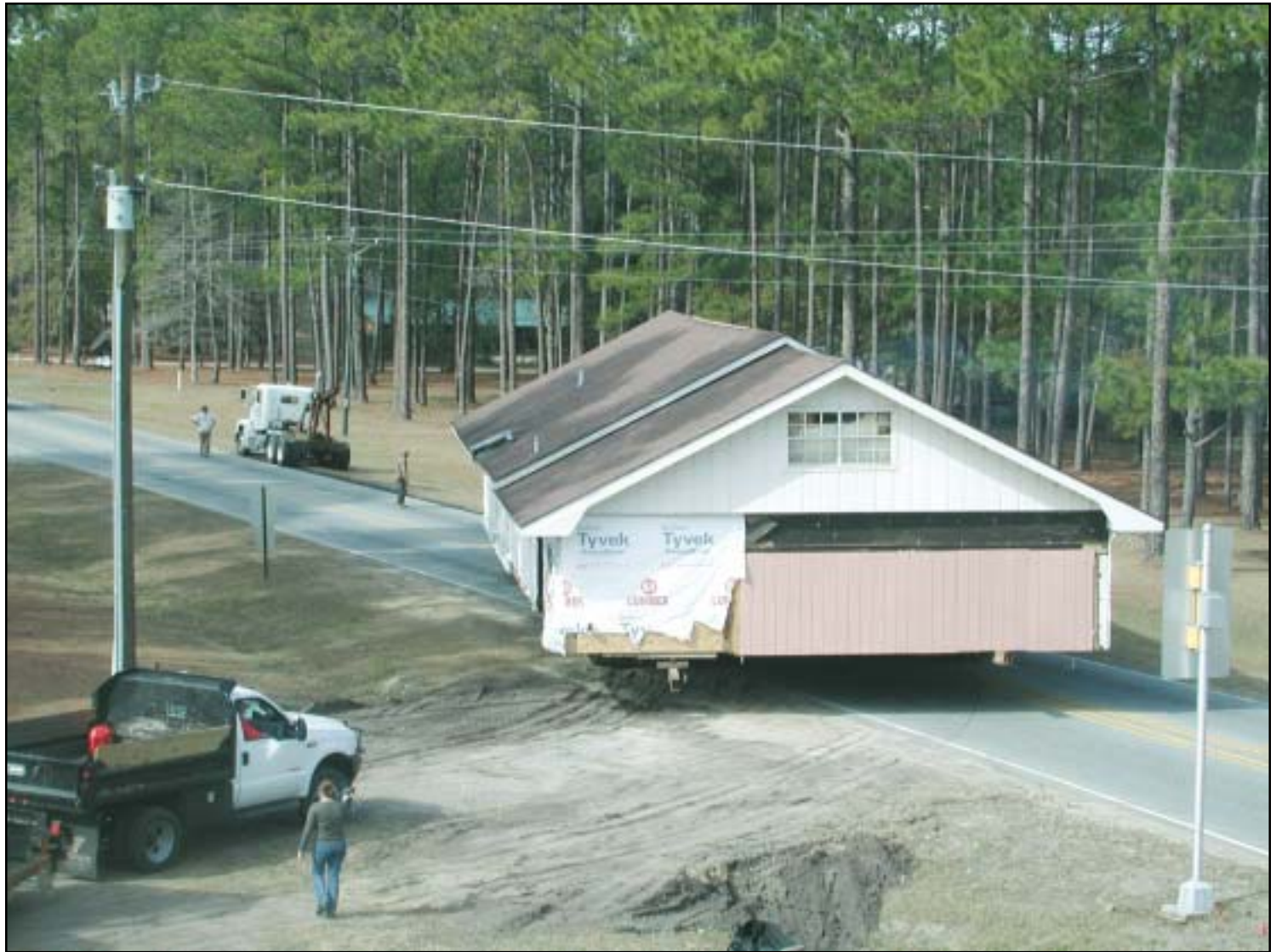
A church on the move: The original worship facility for King of Peace, Kingsland, is on its way back to being a family home in order to make room for the congregation's new building.
